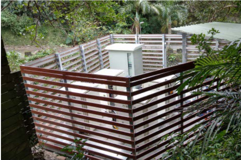
H2 generator with 20 kW FC as UPS for mobile station.
