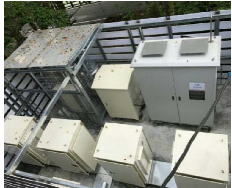
H2 generator @20 NM 3 /hr with 20 kW FC to back up telecom facilities.
