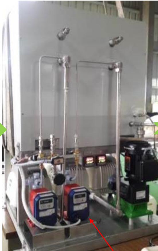
control elements & pipe line
